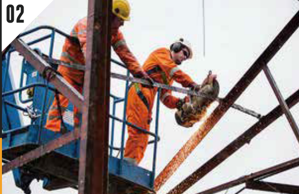
僭建物清拆 - 屋宇署命令 Clearance of Unauthorized Structures
